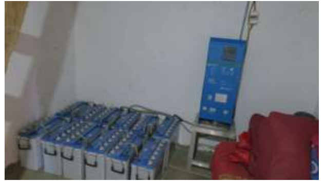
Solar equipment's at Birthing Centre at Bhadgau, Jumla
